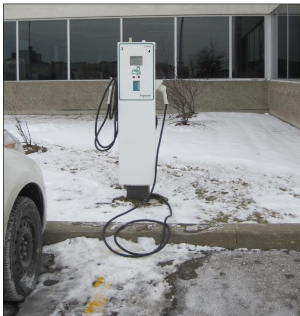
Exhibit 3.1: Typical Electric Vehicle Charging Station
