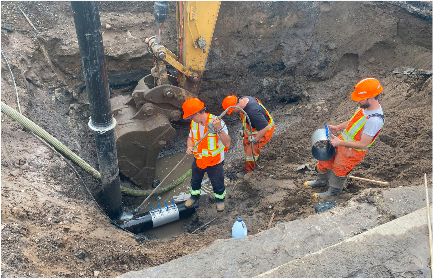
Water Distribution staff, Chris Bruno, Reg Defeo and Bob Gashinski repairing a watermain.
