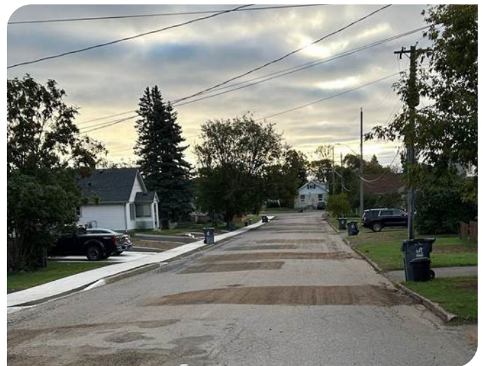
Street showing multiple lead service connections replaced from property line to the watermain.
