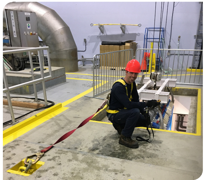
Keith Erickson - Water Treatment Plant Millwright, using a crane to move membranes that are being replaced through the floor.
